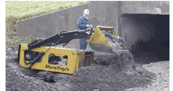
Eliminate Confined Space Issues
